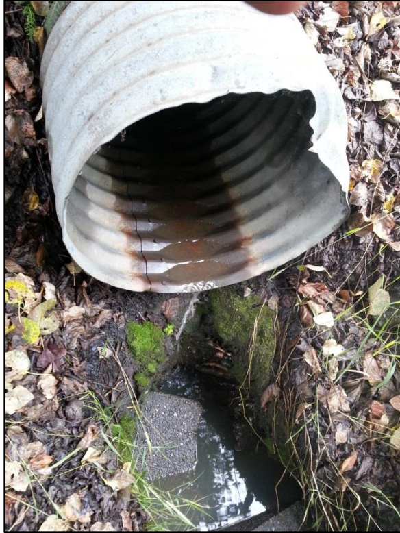
Photograph 7. Outfall SWM07 (484-1), New Seward Highway at Chester Creek.
