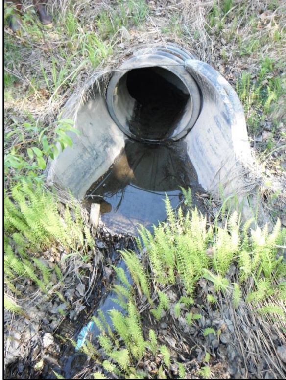
Photograph 1. Outfall SWM01 (1040-3), Ridgemont Drive.
